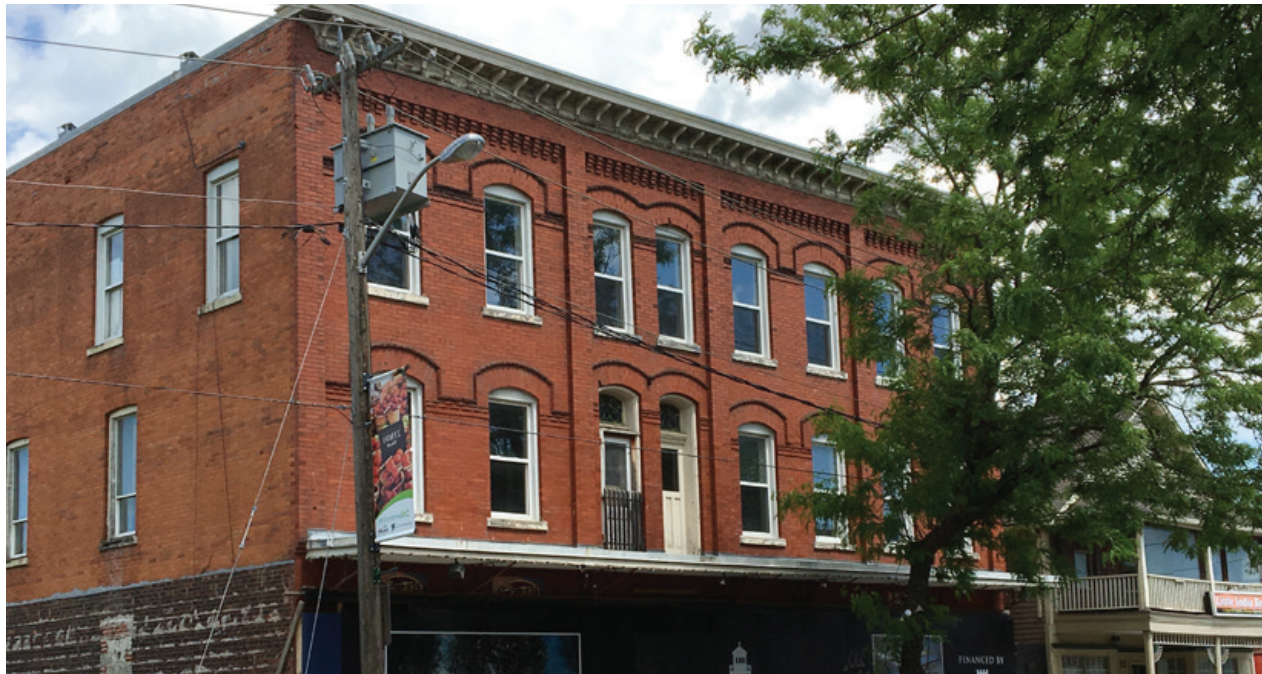
Handsome wood cornice on former hotel building provides protection for masonry and is one of only a few cornices that survive on the Italianate style commercial buildings in Port Dalhousie.
