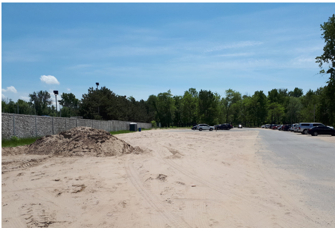
Sand migration near north parking lot
